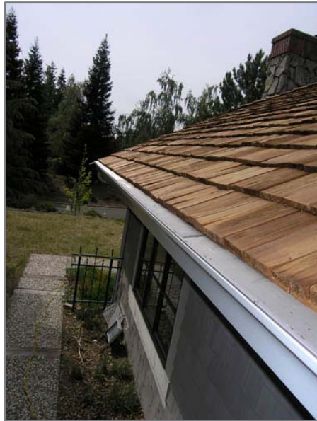
Wood shingle roof with a "Gutter Glove" leaf and debris screen Courtesy of Gutter Glove
